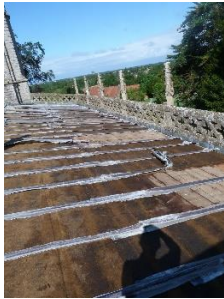
Pictures of roof after lead theft
