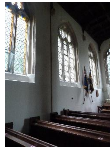
Water damage to the church (stained wall)
